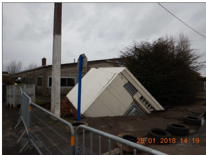
Figure III.21: Effondrement route de Tilloy. Source: DDTM62
