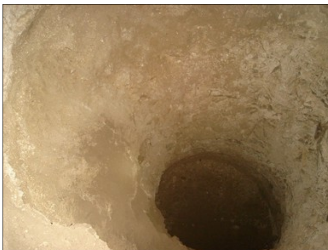
Figure III.19: Rupture de bouchon de catiche rue Émile Zola. Source: GRIMP (ARR285)
