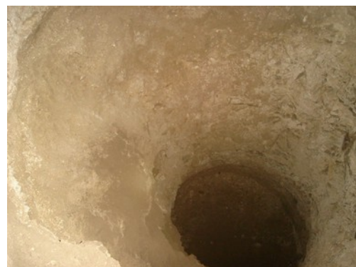
Figure II.9: Rupture de bouchon de catiche rue Émile Zola. Source: GRIMP (ARR285)
